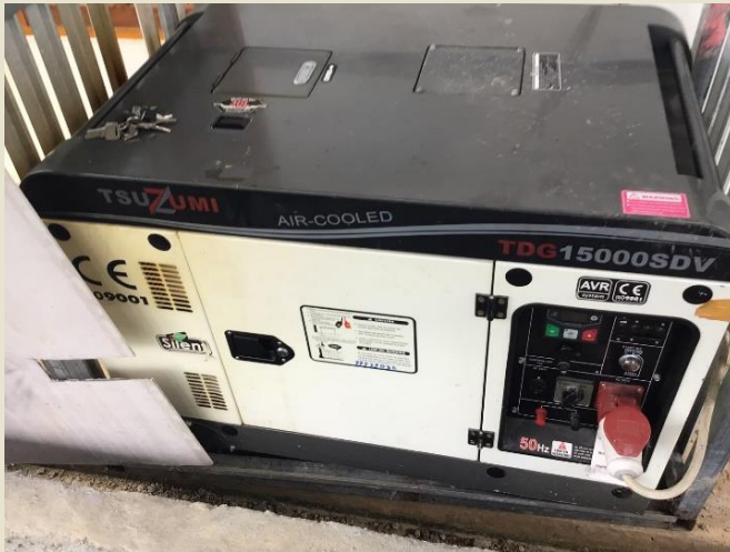
Generator (installed) – St Paul's School, Turiscai
